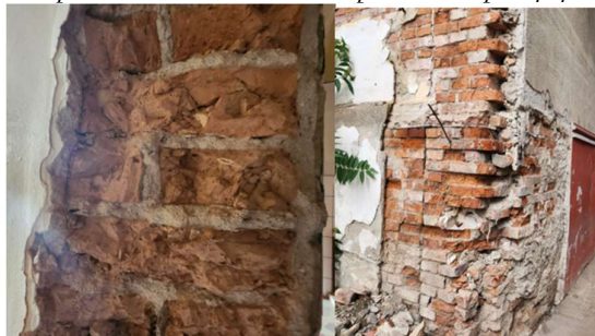
Figure 1. Degraded brick masonry and plaster
